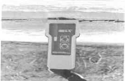
Exterior wall at living room- WME 79.4%
