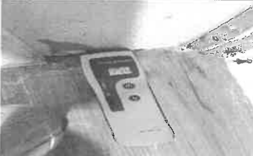
Laundry/ utility room- WME 11.4% at wall next to exit at base
