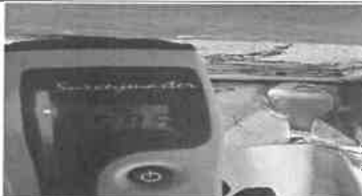
Laundry/utility room- WME 59.6% at wall behind washer & dryer
