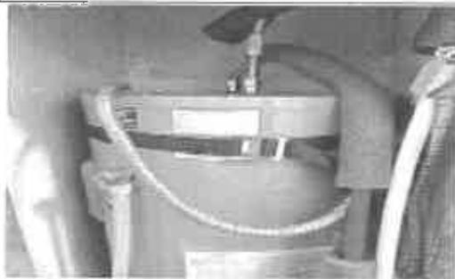
Newly replaced hot water tank in laundry/ utility room
