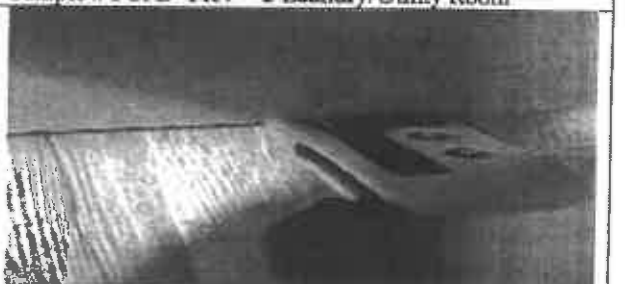
HVAC area with red alarming moisture content
